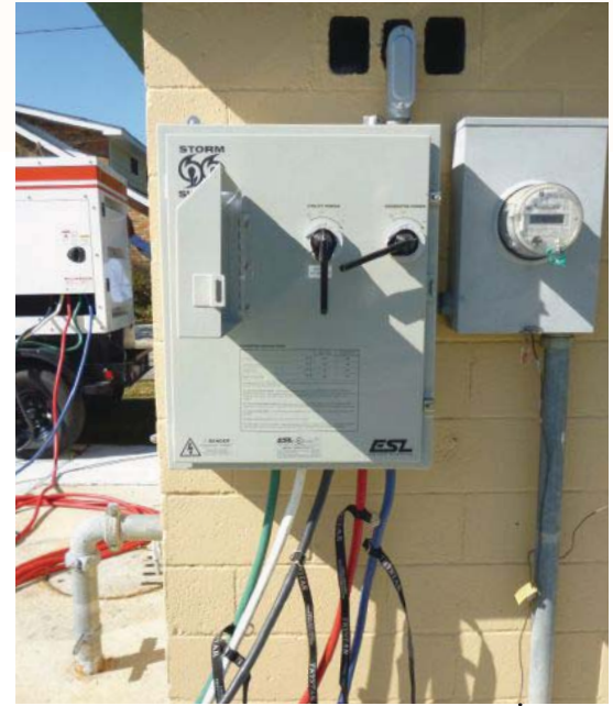
Figure 2: With the help of a portable generator, this MTS provides emergency backup power to a business.
