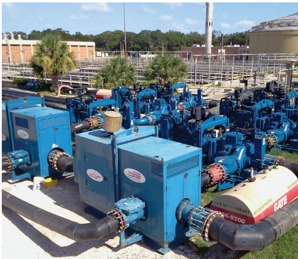
A sewer bypass at the Buckman Waste Water Treatment Plant in Jacksonville, FL
