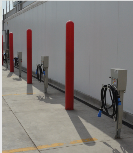
Single Gang Shore Power Outlet 50A 240VAC ESL Series: 2223-73B
