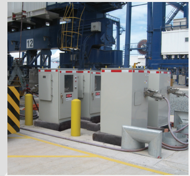
ERTG Disconnect Cabinet 3300V 125A 50Hz ESL Series: 5100-46B
