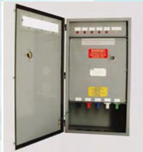
400A Cam-lock Style Distribution Unit
