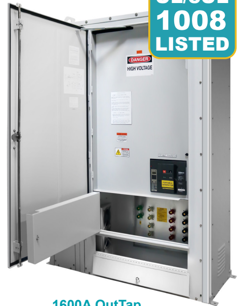
1600A OutTap with Breaker
