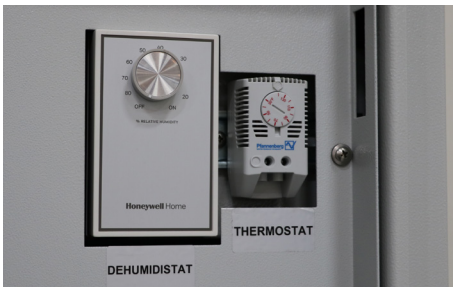
Thermostat, de-humidistat and heater
